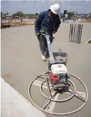
Above: A Bondfield Construction worker smoothes concrete atop a newly poured floor.
